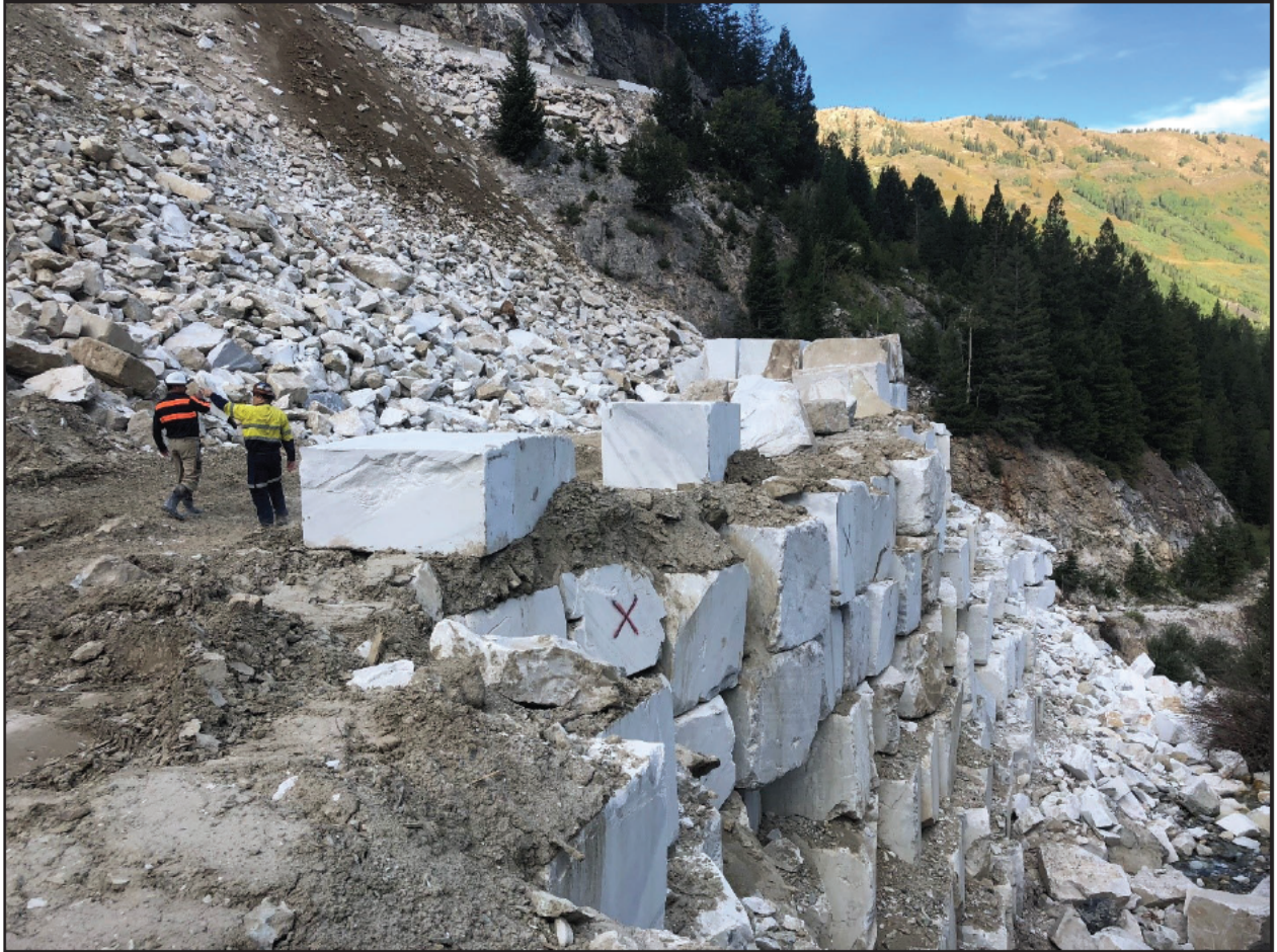
Figure 6. Example of marble block stacked to create a retaining wall. View to the northwest; photo captured August 30, 2018.
